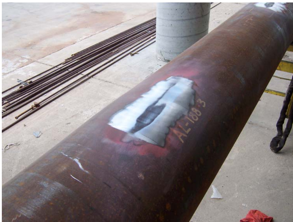
Figure 4 - Gouge removed by grinding
